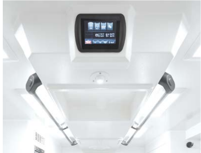
The ceiling centre is used to contain medical equipment, energy and oxygen supply as well as the touch screen used to control the ambulance table and the heating/air conditioning system.
